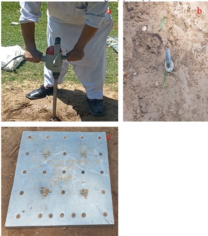
Figure 3: Test setup, (a) drill machine, (b) installation of piles, (c) screwing of pile.
